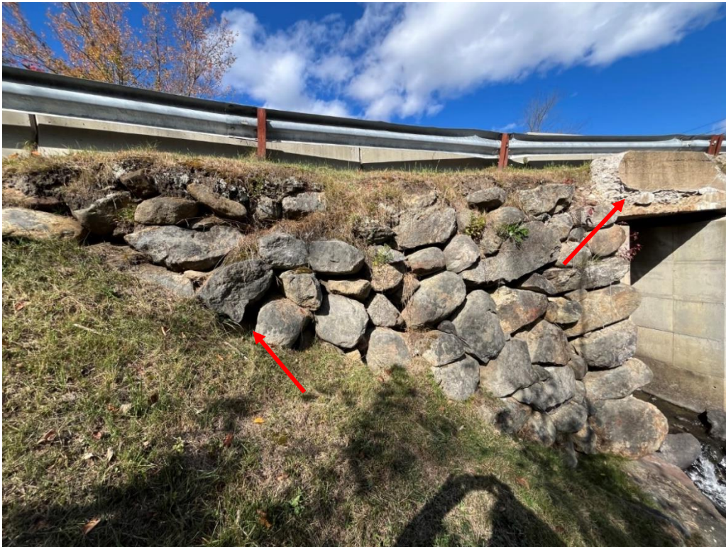
Photo 8: Downstream side of dam near right abutment contact. Note – voids in dry-stone masonry and spalling of concrete roof section.
