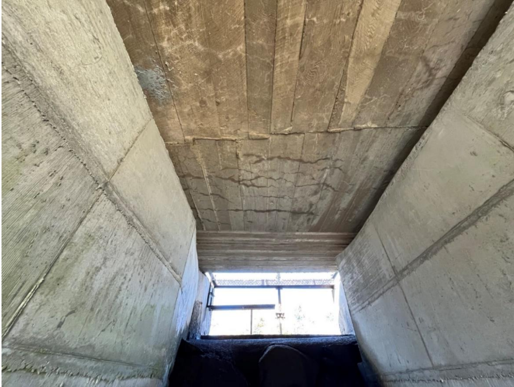
Photo 11: Top view of concrete side channels and roof deck (supporting crest roadway) downstream of low-level outlet discharge pipe.
