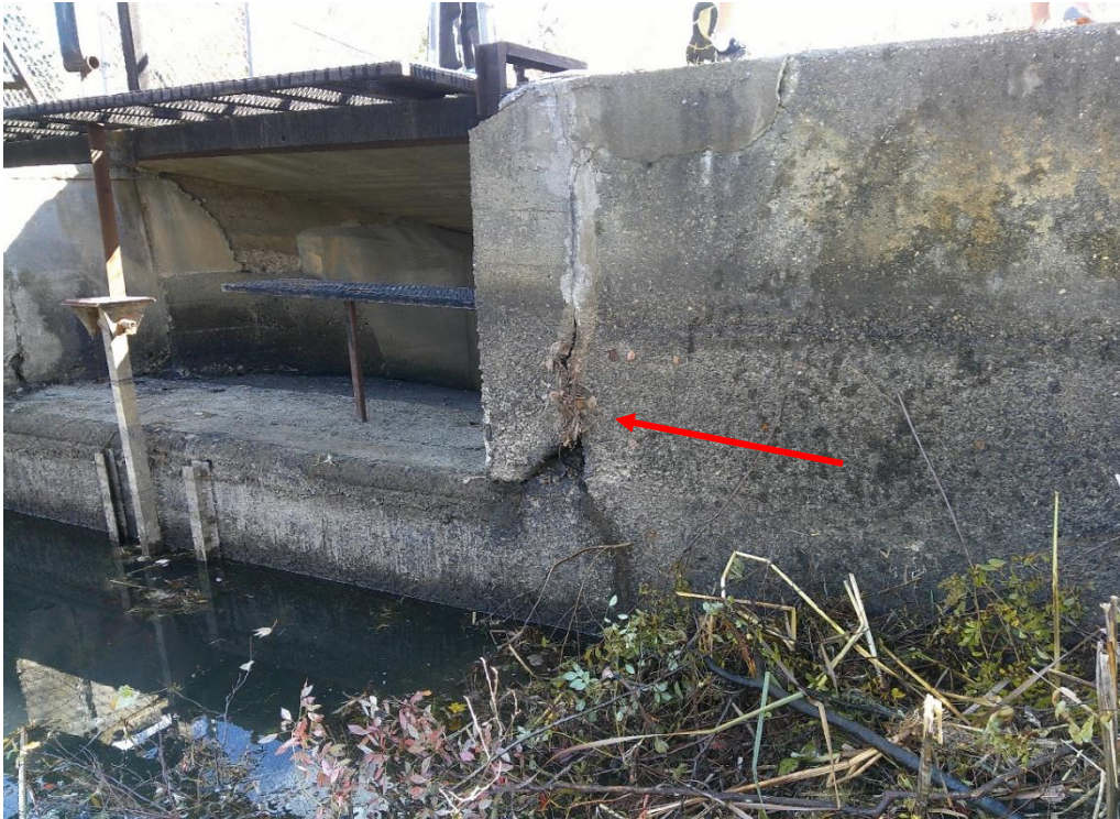
Photo 3: Upstream concrete wall at spillway. Note cracking/spalling at spillway inlet area.
