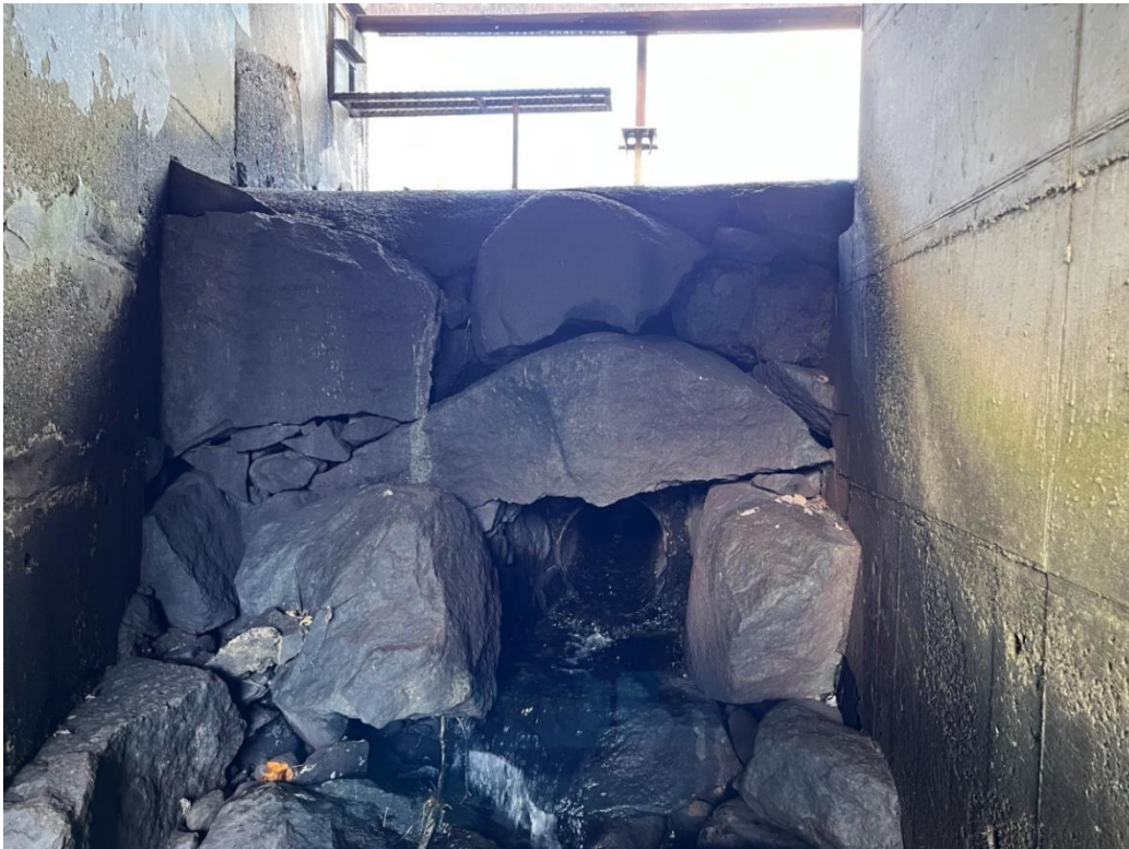
Photo 6: Downstream end of 18" diameter low-level discharge pipe at the downstream side of concrete faced portion of the spillway.
