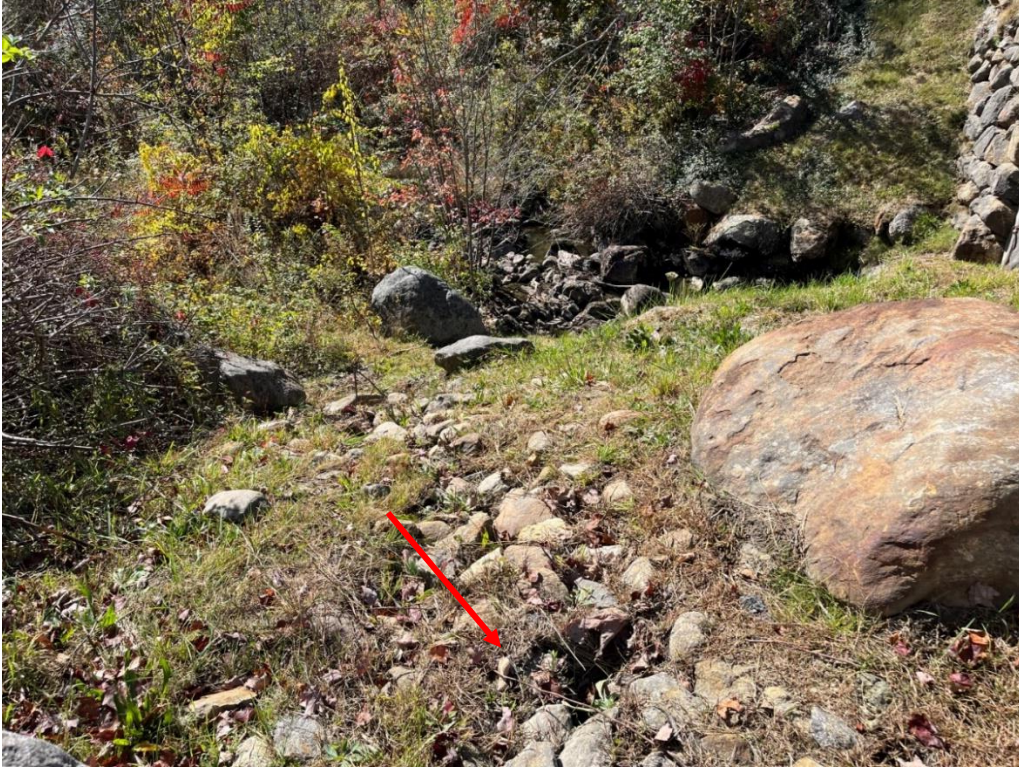
Photo 9: Erosion from road runoff in the stone-lined channel in the left downstream embankment portion facing downstream.
