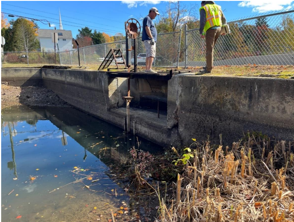
Photo 1: Upstream side of dam. Note spillway intake and low-level gate at center.
