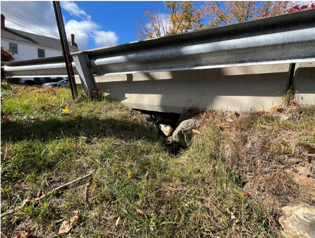
Photo 10: View of depressed/eroded area beneath/downstream of the “jersey” barrier on the downstream side of the crest roadway. Deficiency caused by uncontrolled surface water runoff.
